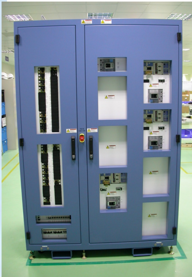
Power Distribution System
